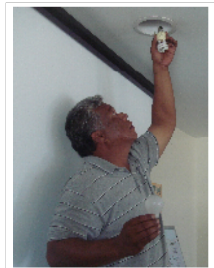
Replacing inefficient light bulb with a compact fluorescent light
