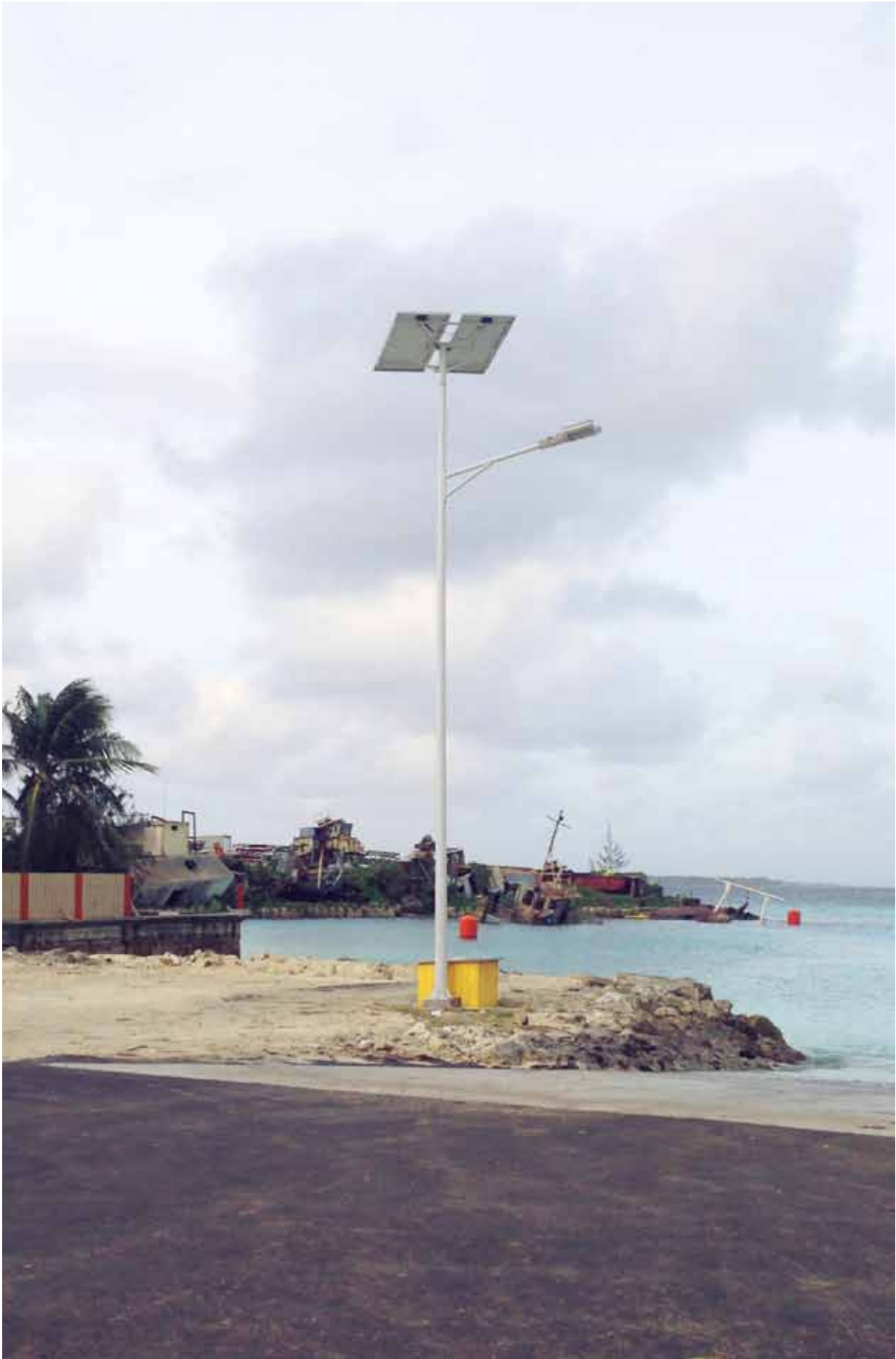
Solar street light Photo: H. Wade
