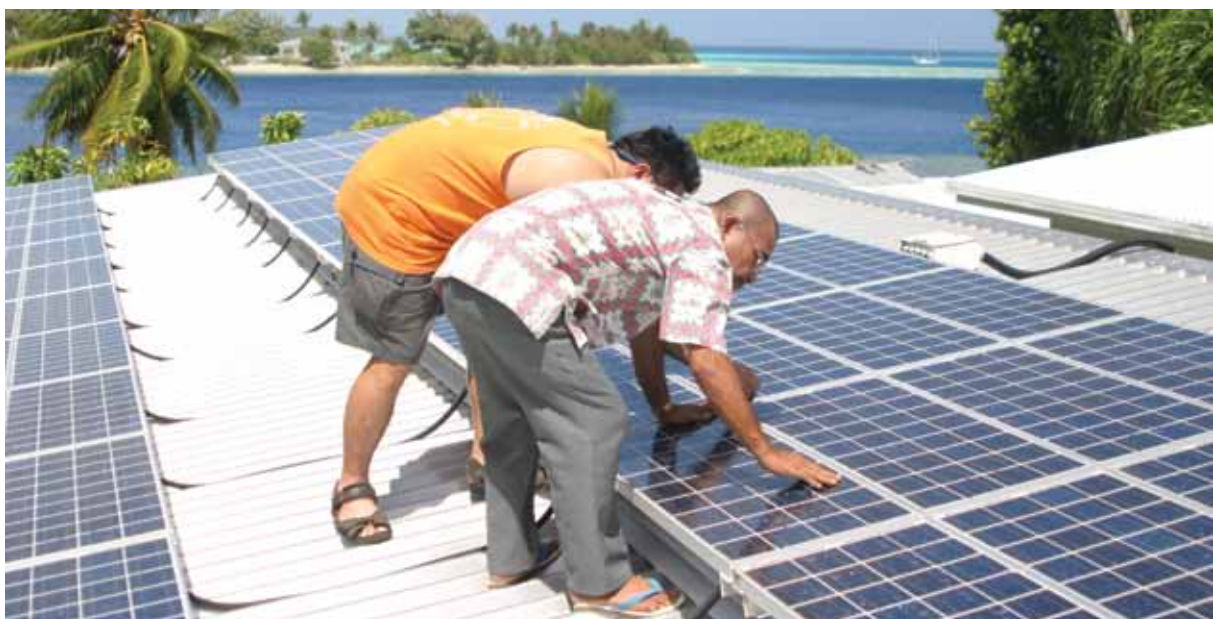
Solar PV for Jica Freezers Photo: H. Wade
