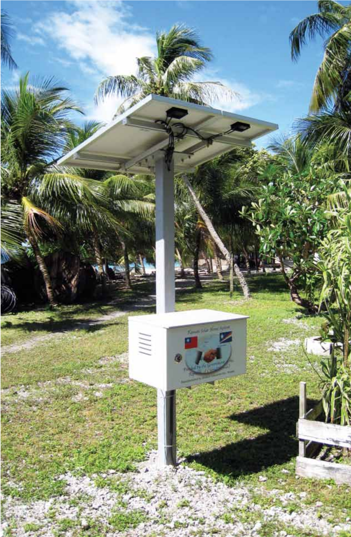
Solar PV street lighting in island community Photo: H. Wade
